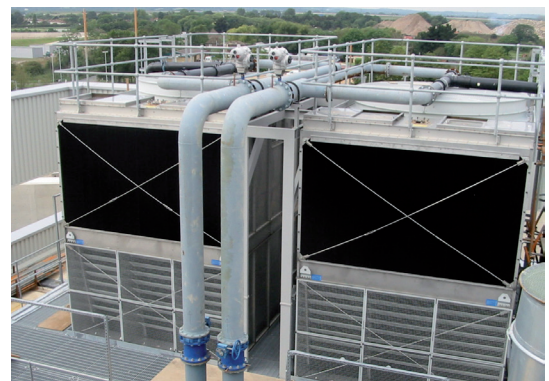
Combined inlet shields retrofitted to the top half of BAC S3000 cooling towers with old style louvres at the bottom
