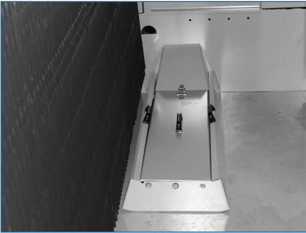
Cold water basin and basin strainer
