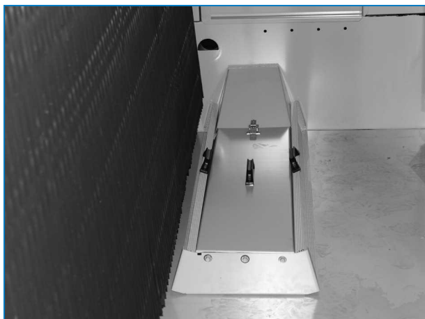
Bazen hladne vode i filter bazena
